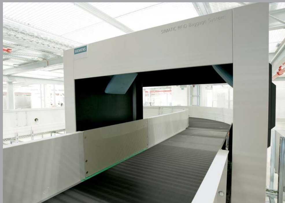
The SIMATIC RFID Baggage System for accurate baggage identification using RFID in the UHF range.
